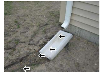
Extensions should be at least 2-5 feet out depending on the grade and available space to distribute water run off.
