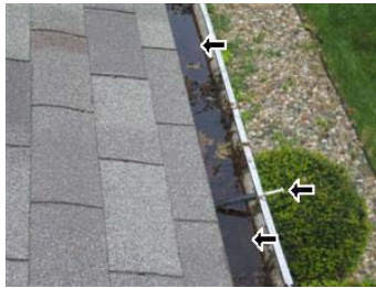
Keeping gutters free and clear of debris at all times is key to a home's drainage system working properly.
