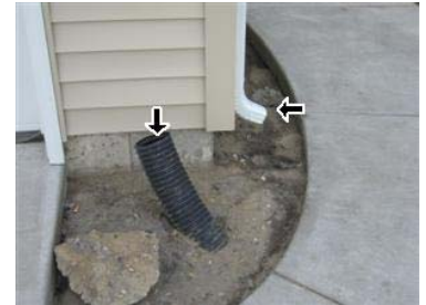
Water is guaranteed to puddle against a home's foundation if downspout extensions are missing and eventually cause water to infiltrate the basement or crawlspace.
